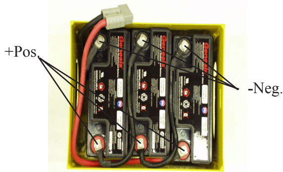
Figure 1. Battery cable and terminals
